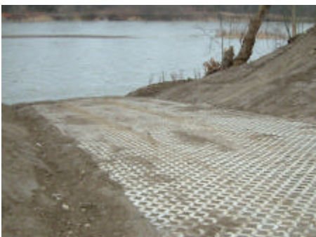
The ramp at Brant Conservation Area is built to accommodate canoes and drift boats that use this portion of the river.
